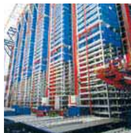
The modern high-bay warehouse ensures efficient logistics
